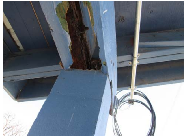
Photo 2 – 8x8 Timber Beam Deterioration
