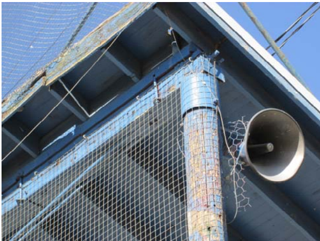
Photo 5 – Opposite End Condition of Beam Assembly
